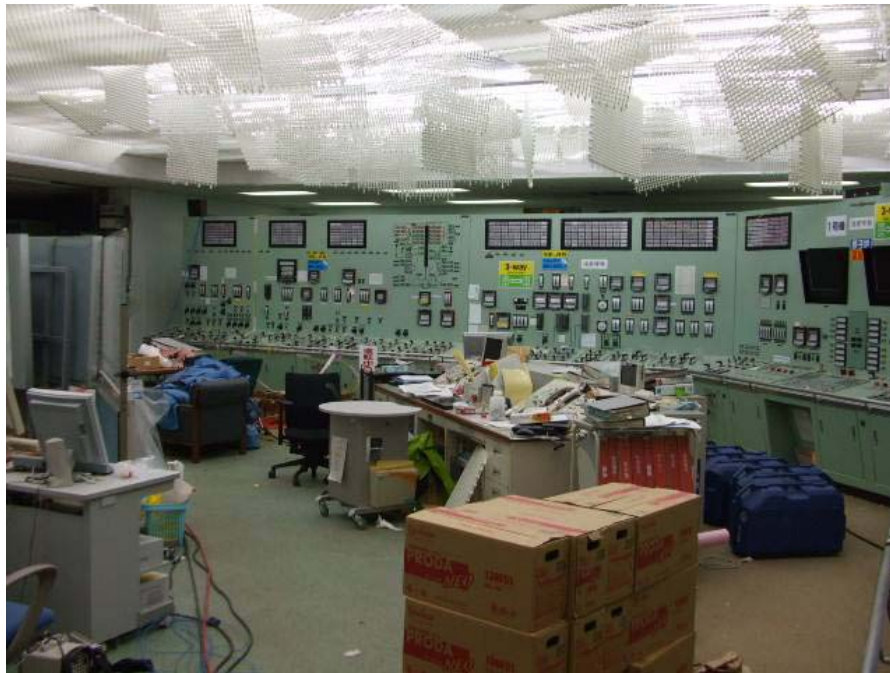
Unit 1 Main Control Room turned on (The light fixture is broken by the earthquake)
